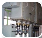
Power sensitive equipment
