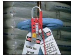
Lockout gate valves
