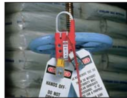
Lockout gate valves
