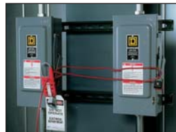
Lockout single or multiple electrical disconnects
