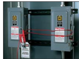
Lockout single or multiple electrical disconnects
