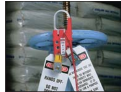
Lockout gate valves
