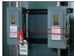
Lockout single or multiple electrical disconnects
