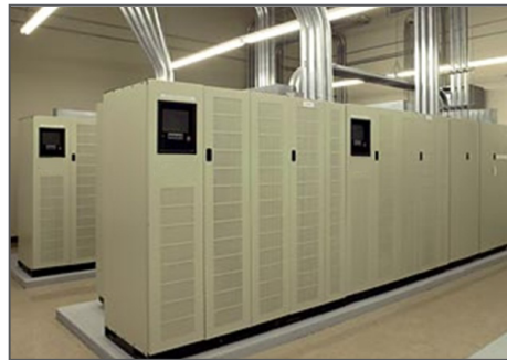
Uninterrupted Power Supplies
