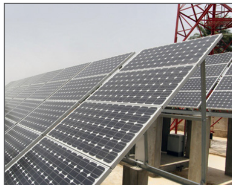
Solar-Powered Cellular Base Station
