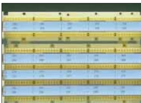
Network Systems Labeling
