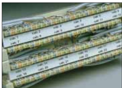
Network Systems Labeling
