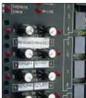
Label switches, relays and other devices
