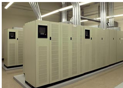
Uninterrupted Power Supplies
