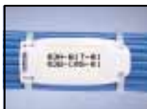
Cable bundle labels
